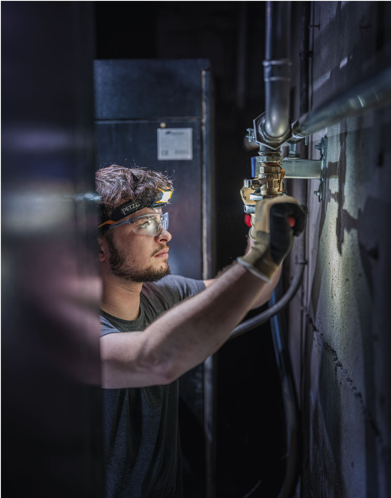
Stainless steel plumbing, France © 2023 Petzl Distribution - Rémi Flament - Croze
